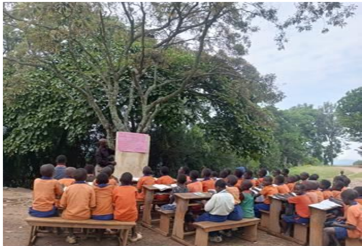
Kihungu Primary School classroom block had its roof blown off. Learners are currently studying under trees
